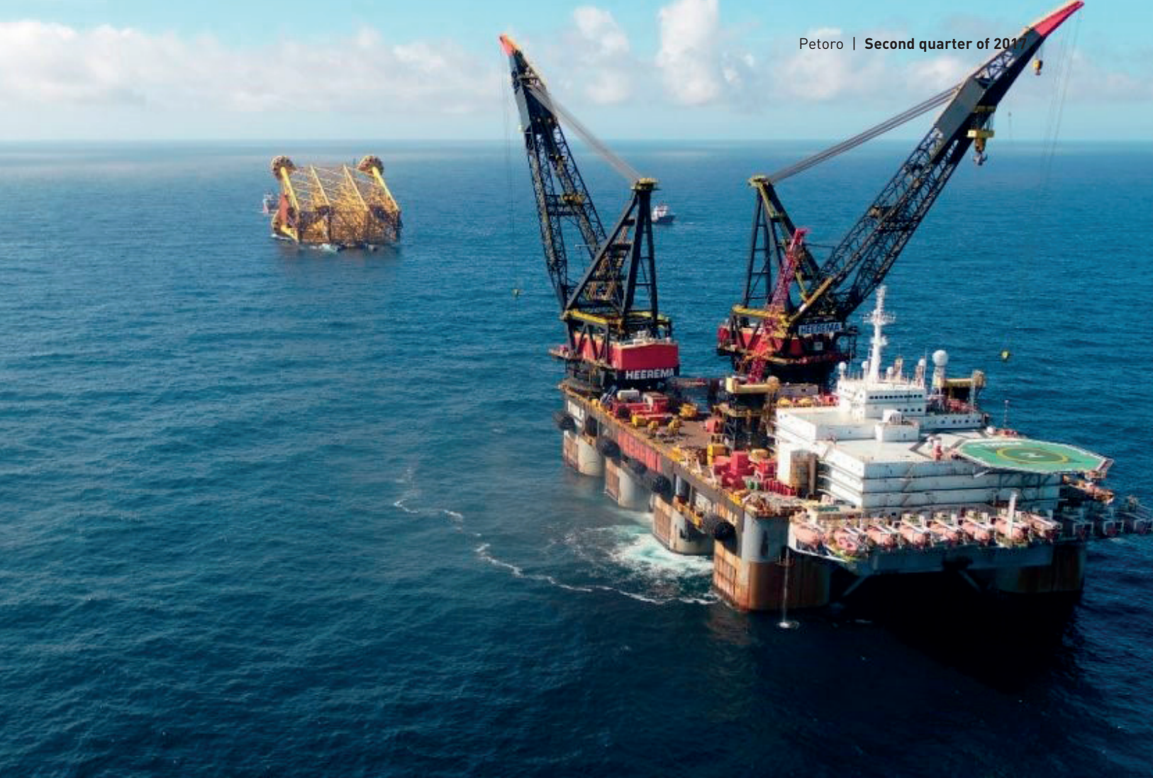
First visible sign of the Johan Sverdrup field in the North Sea. The jacket for the Johan Sverdrup riser platform is being installed. Source: Statoil
